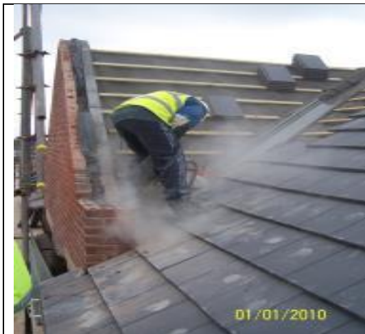
Slaba praksa – rezanje strešnikov brez nadzornih ukrepov (National Federation of Roofing Contractors Ltd, GB)
